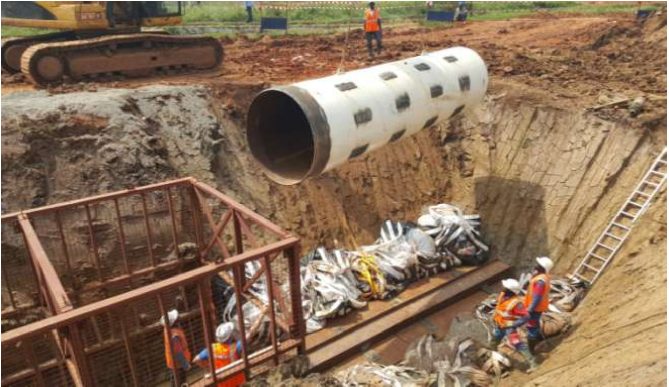
Pic. 3: The first steel pipe \varnothing 1'500 mm (59") is lifted into the ramming pit.
