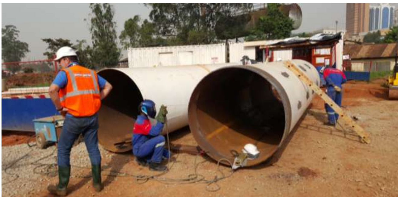
Pic. 1: Preparation of the cutting ring for the first steel pipe. It reinforces the „nose“ of the steel pipe.
