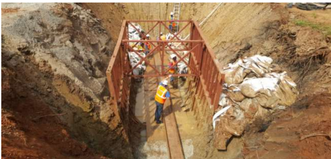
Pic. 2: Preparation of the ramming pit. A U-Profile is installed with the correct alignment. The U-Profile guides the steel pipe.
