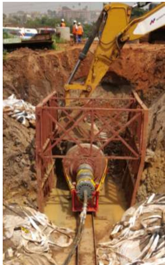
Pic. 5: The steel pipe ram is assembled and connected to the steel pipes. The excavator shovel holds the steel pipe during the first meters.
